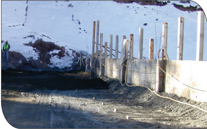
View of upstream facing formwork during construction. Note water stops and steel rods anchoring the concrete facing to the RCC
