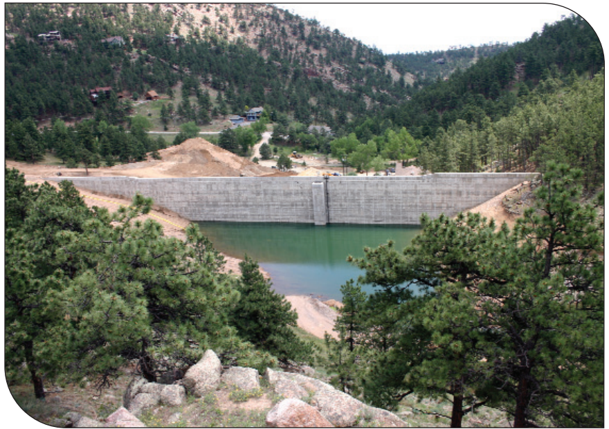
A view looking at the upstream face of the dam during initial filling
