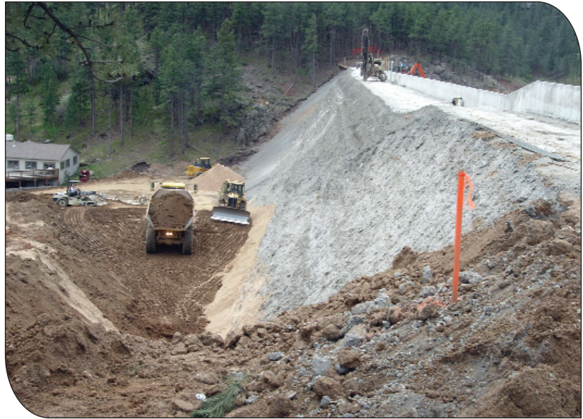
A view showing crest of dam, parapet wall, and unformed uncompact downstream face
